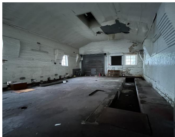
Figure 27 Interior of the substation facing northeast.
