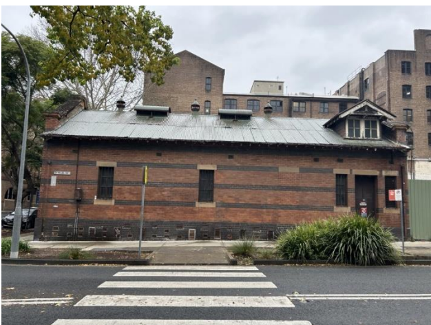
Figure 26 View south detailing the northern elevation of the electricity substation.
